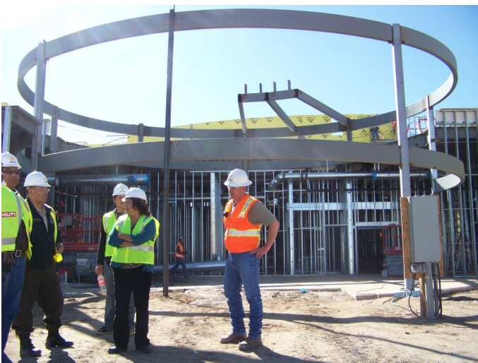
The Law and Order Committee tours the construction site for the Crownpoint justice/public safety facility.
